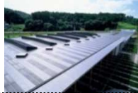
Example of installation of solar energy system (Koriyama City, Fukushima Agricultural Technology Centre)
