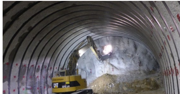
The Sekiba Tunnel in the Kawamata Town section on the National Road Route 114 was opened on 2 Mar. 2022
